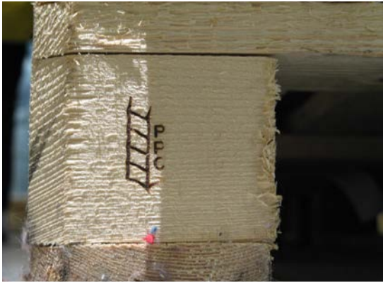
Mark is incomplete
